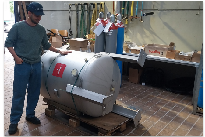
Part of the water injection system at University of Mons. Source: UMONS.
